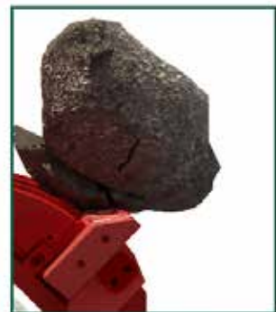
Worn out blow bar
